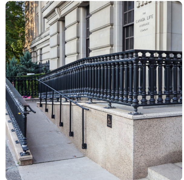
A ramp in a compatible style was added to the Sun Life Building, Toronto, Ontario
